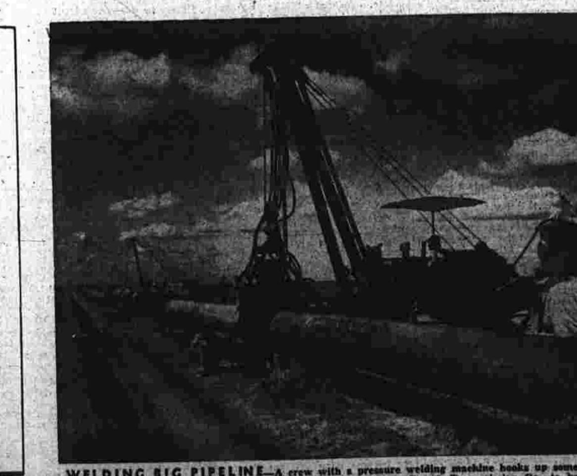
WELDING BIG PIPELINE —A crew with a pressure welding machine works up some of the Texas sections of the 1,265-mile pipeline of the Tennessee Gas & Transportation Co. to bring natural gas from Coaling, Texas, to Charleston, W. Va.
